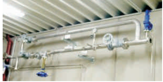
Pressure reducing station
